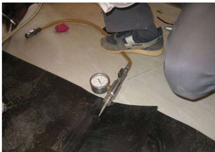
Figure 4.16: Proof of welding seams
