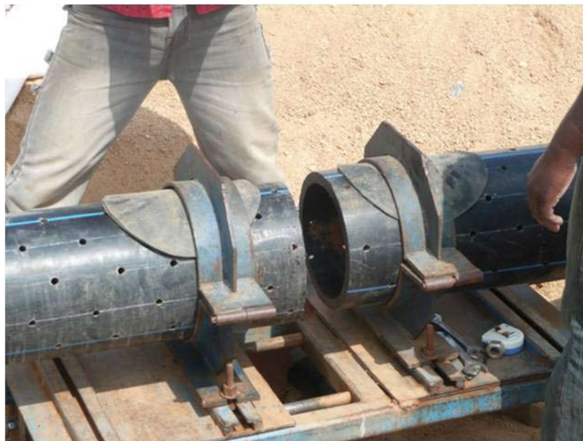
Figure 4.18: Proper Holed Leachate Pipes
